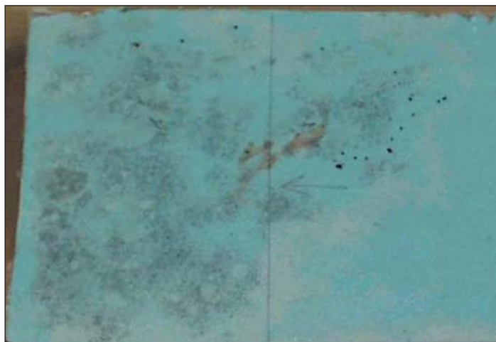
Sample 2: This water-resistant drywall showed moderate mould growth.
